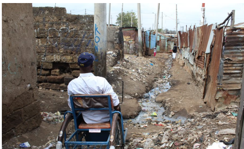
Example of the impact poor drainage and sanitation has on roads in informal settlements
