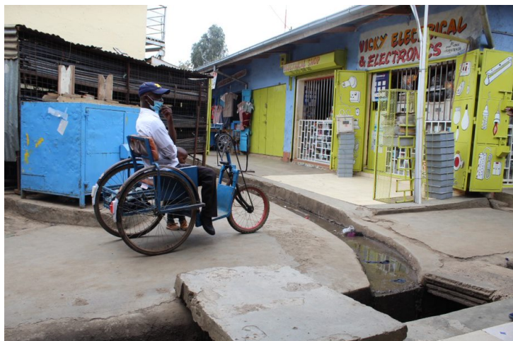
Example of poor drainage planning blocking routes to amenities
